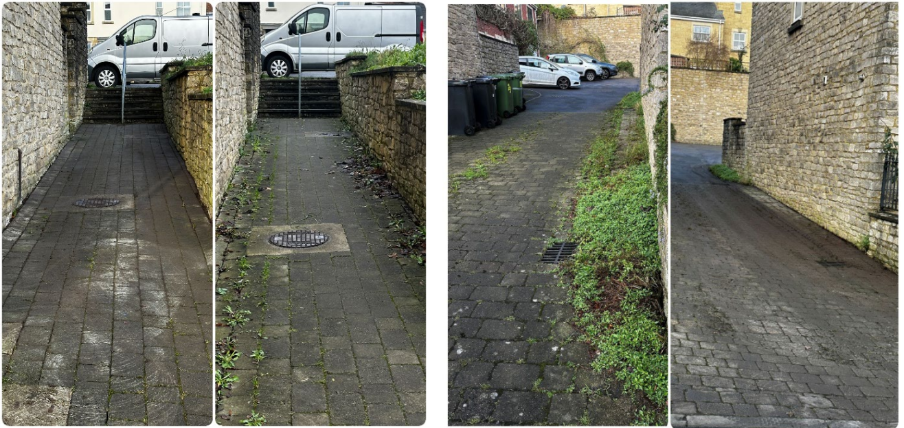
Figures 15 and 16 - Before and after of two lanes cleaned near Waterloo. The street with the dense weeds (righthand pictures) would have taken several hours to clear with the existing technique. The sweeper took approximately 20 minutes.
